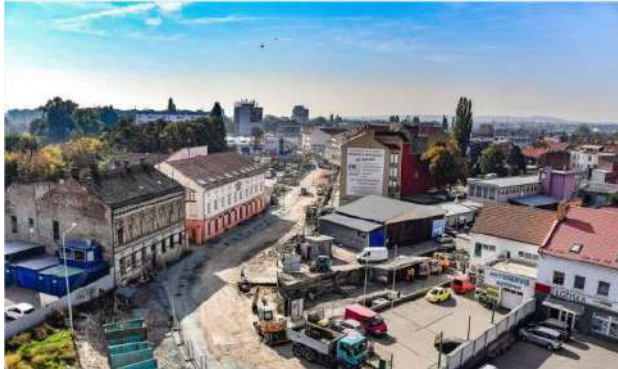
New district Trnitá - transport and technical infrastructure (modernization of the bus station Zvonařka, tram Plotní, replacement of steam pipelines for hot water pipelines)
